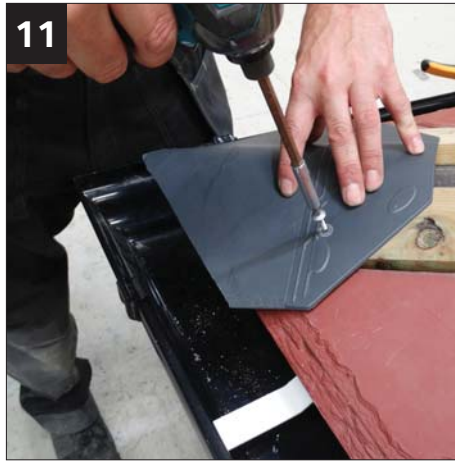
11 Cut along the lines on the hip tile and fix to the battens on the hip.
